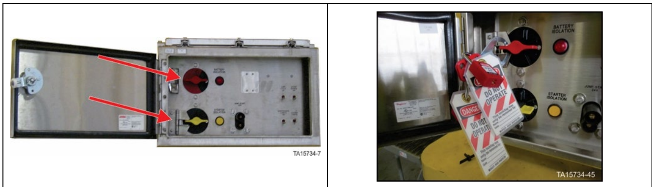
Battery Isolation Box – Battery isolation switch in OFF position with locks in place
