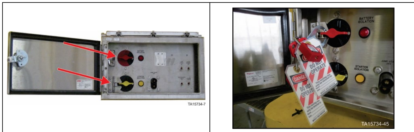
Battery Isolation Box – Battery isolation switch in OFF position with locks in place
